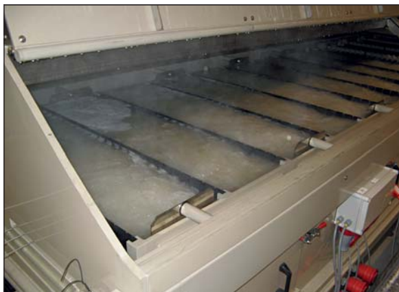
View of cleaning plant
